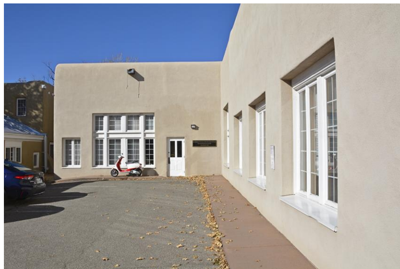
Photo 7: South and east elevations, 1942 building. Infilled overhead door opening at center. Camera facing west.
