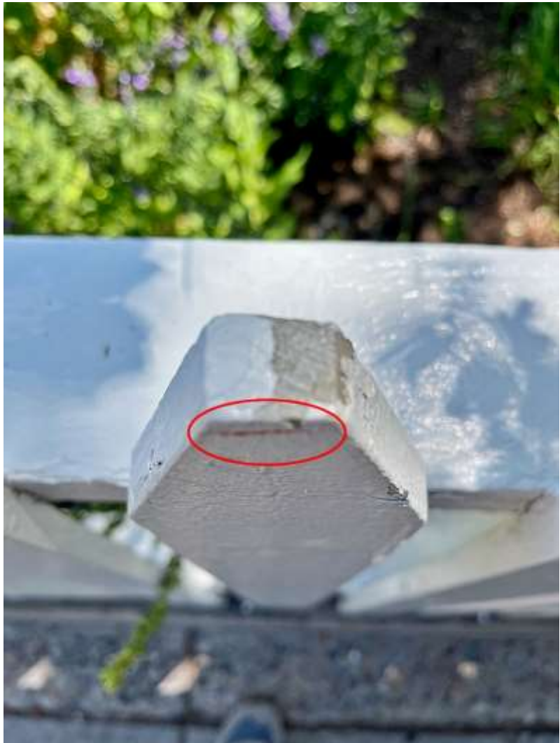
Figure 4: Picket head. Apparent cut line circled. July 25, 2023, John W. Murphey.
