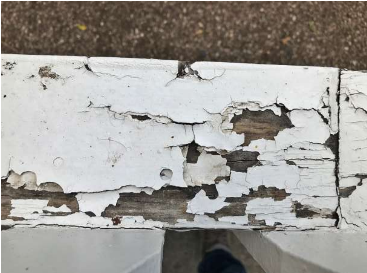
Figure 8: Top rail with multiple layers of paint. July 2, 2021, John W. Murphey.
