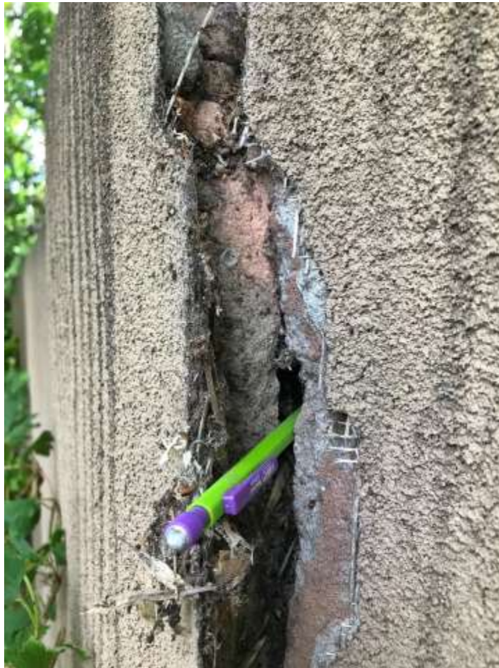
Figure 24: Delamination of “Middle Section,” showing multiple stucco applications. July 2, 2021, John W. Murphey.
