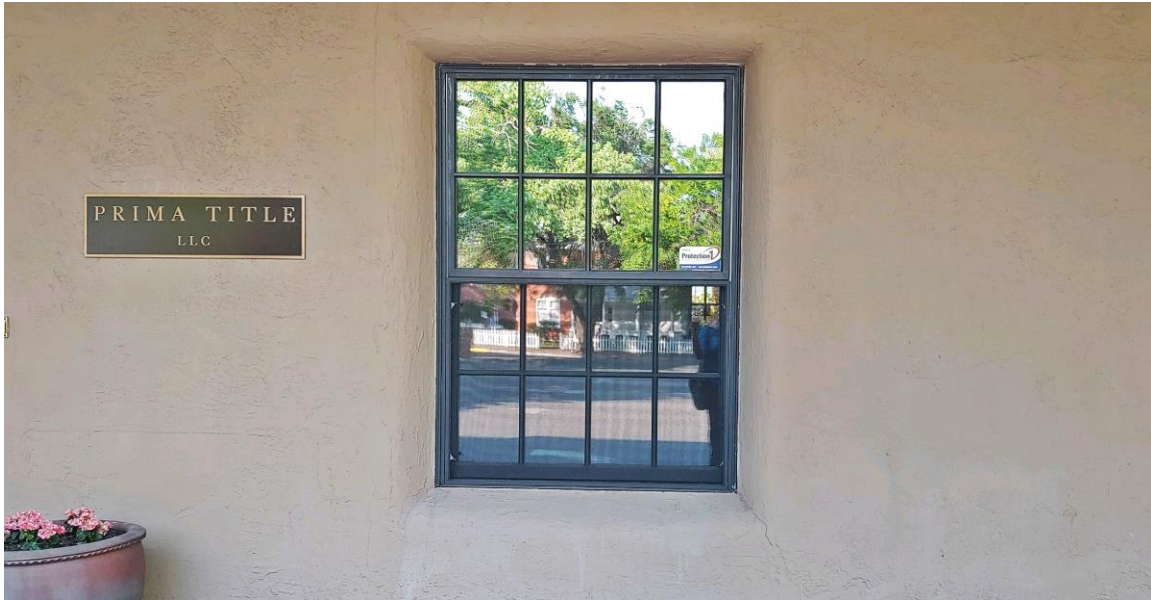
Photo 5: West façade. Typical clad window found throughout building. Camera facing east. Robyn Powell: June 13, 2021.
